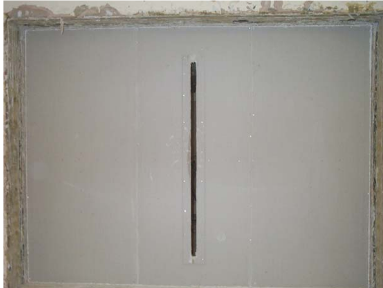
Figure 6 Empty slot, receive room side
